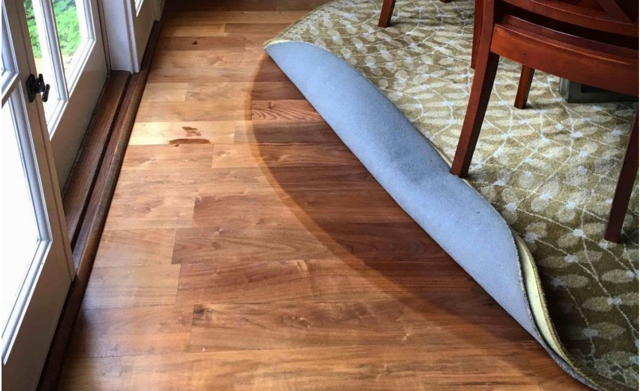
Sun-bleached hardwood floor from having direct sunlight through the house window. 19
